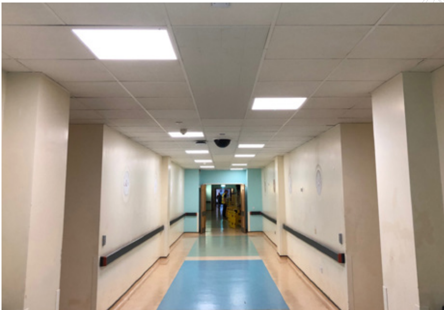
After Energys LED upgrade
